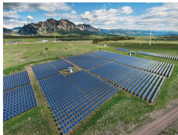
A solar array and wind turbine at the National Wind Technology Center in Jefferson County, Colorado Dennis Schroeder/NREL
